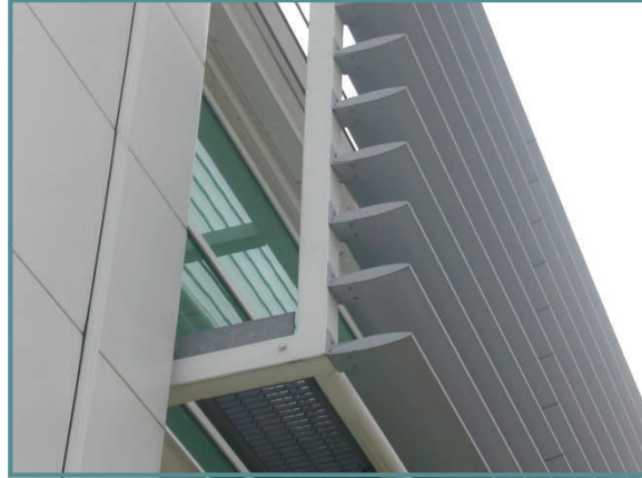
In built walkway for window cleaning
