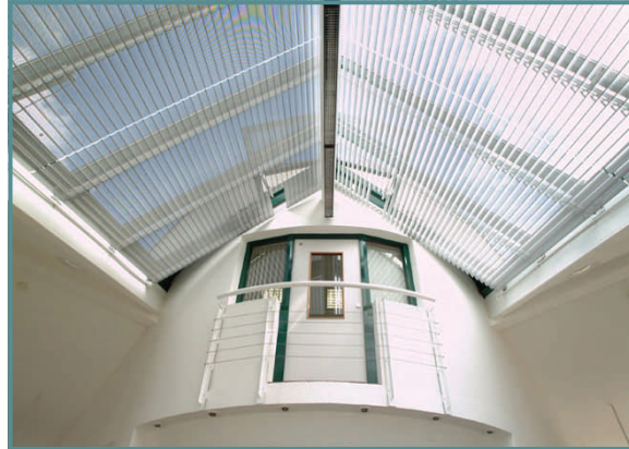
Blinds in open position
