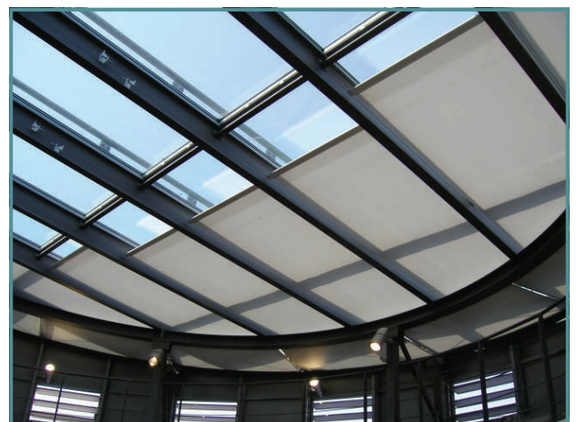
Drum atrium blinds partially deployed
