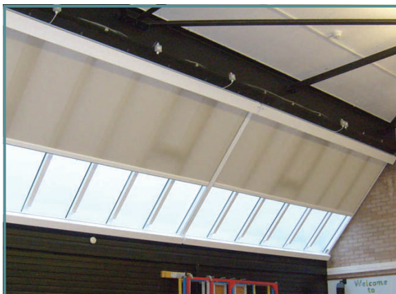
Roof blinds partially lowered
